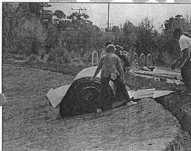
In July the teens installed an 8,723 square foot pond liner which will make
